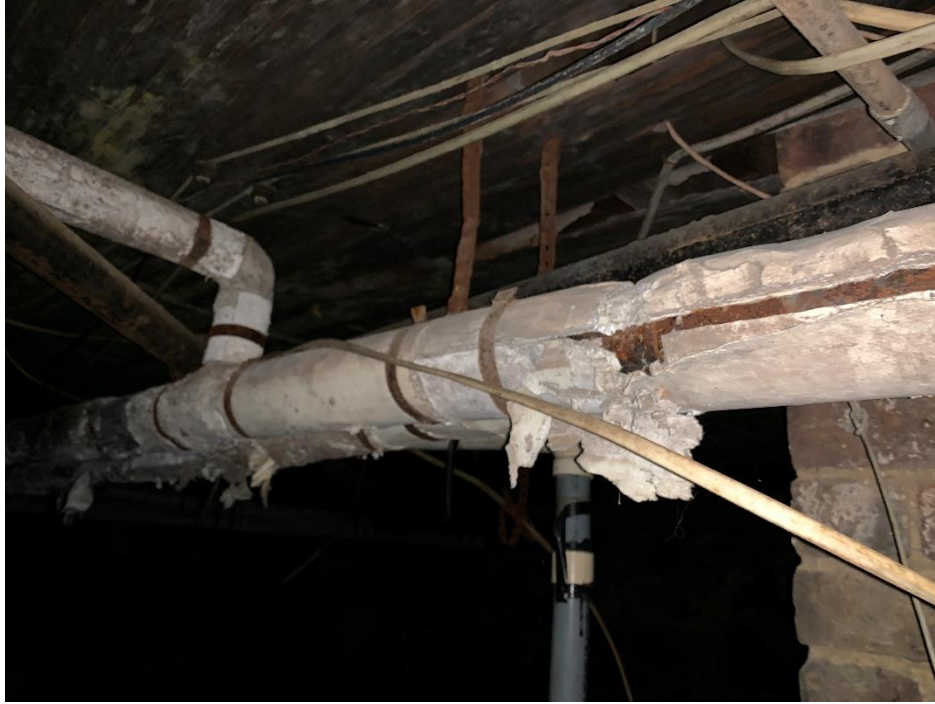
View of asbestos containing air cell pipe insulation located in the basement of the structure
