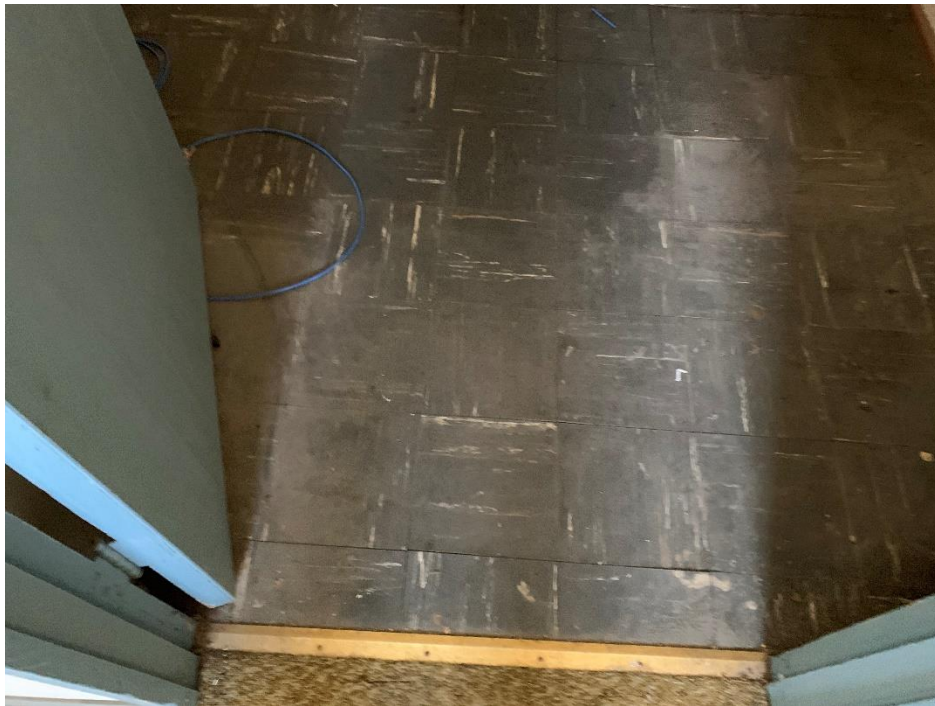
View of asbestos containing 9x9 Floor Tile in the first floor bathroom 1
