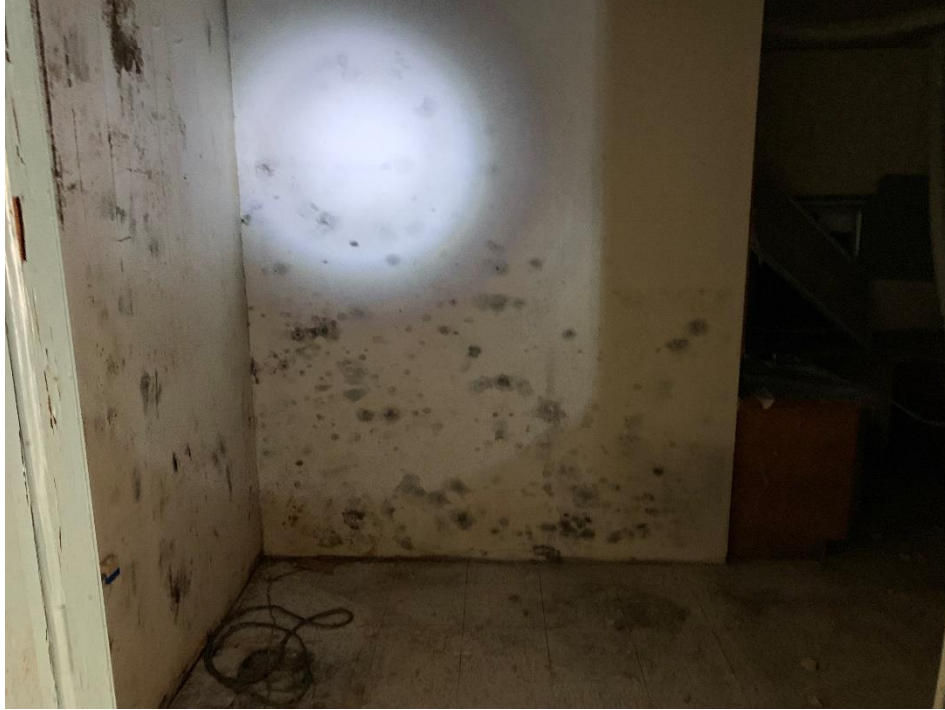
View of mold growth on wall of magistrate office
