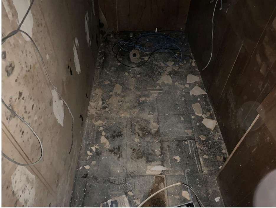
View of asbestos containing 9x9 vinyl floor tile in the magistrate office
