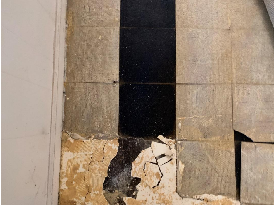
View of asbestos containing 9x9 vinyl floor tile located in the hallway of the second floor underlying carpet
