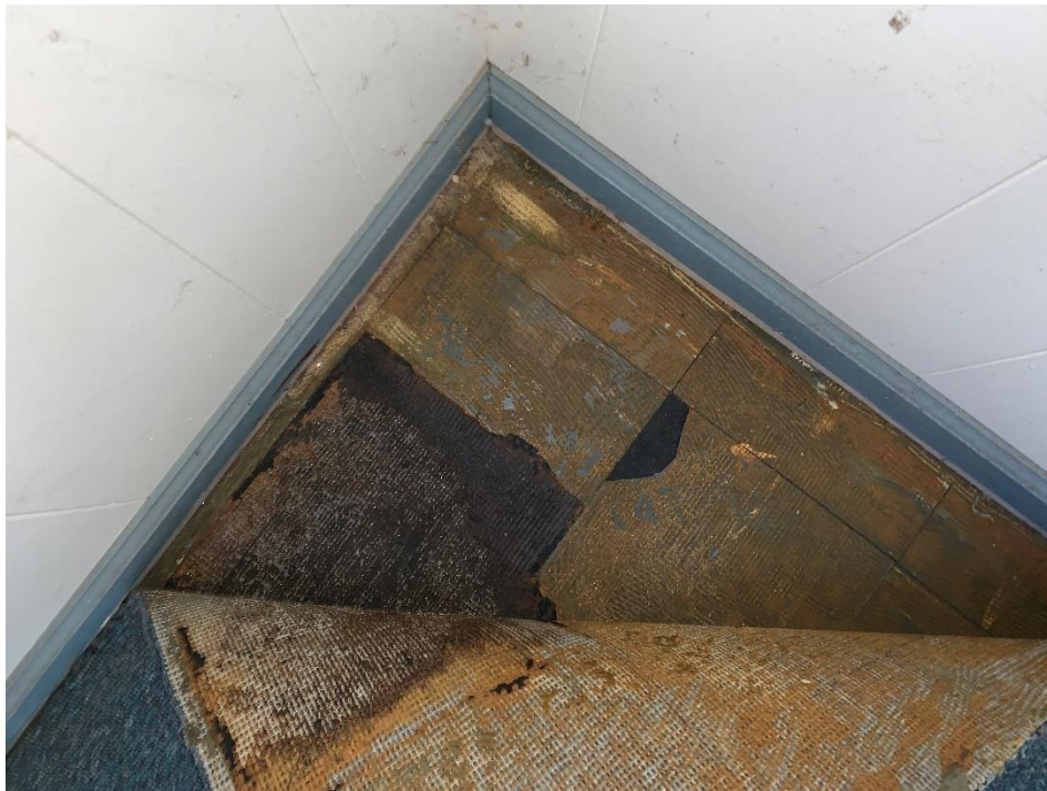
View of asbestos containing vinyl floor tile which underlies carpet in office 4 of the first floor
