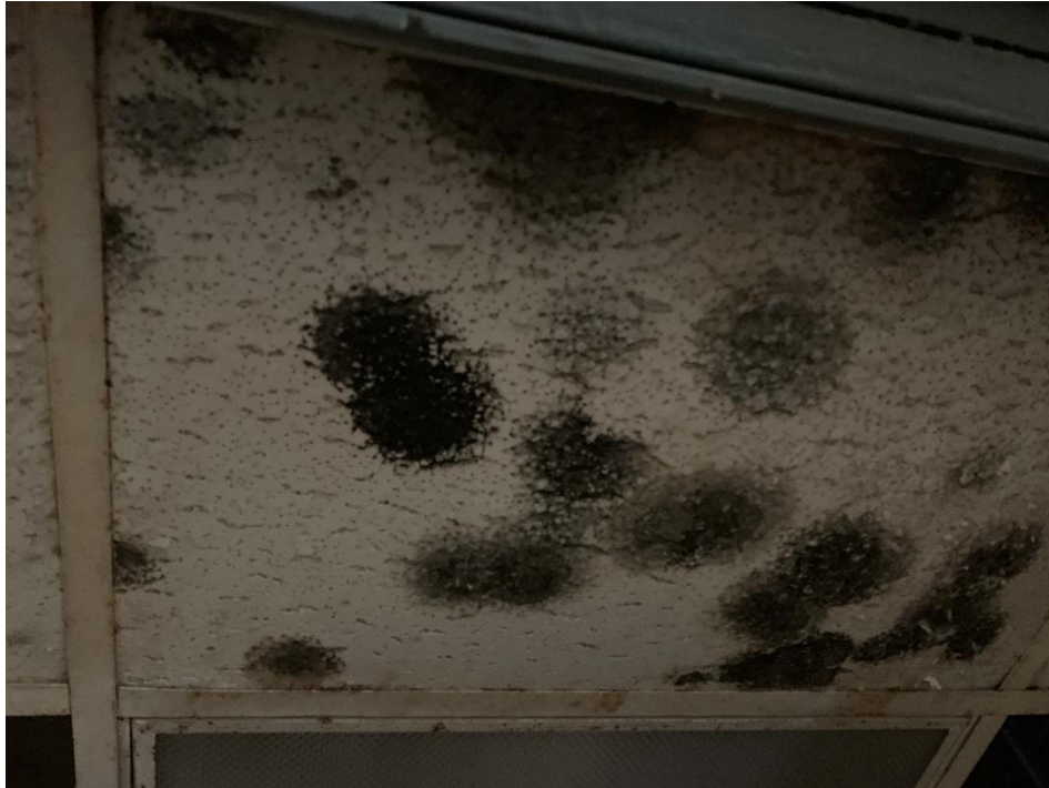
View of mold growth on ceiling tile of magistrate office
