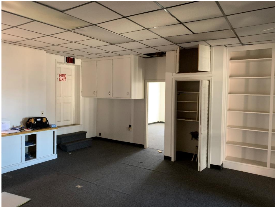
View of the second floor lobby. Note that asbestos containing sheet vinyl backing was identified underlying carpet and fiber board
